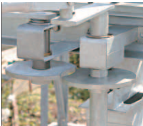
Both Main and Earth Switch Open
